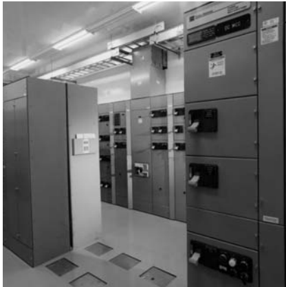
Interior of Integrated Power Assembly
