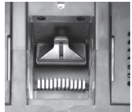
Magnum DS Breaker Contacts (Arc Chutes Removed)
