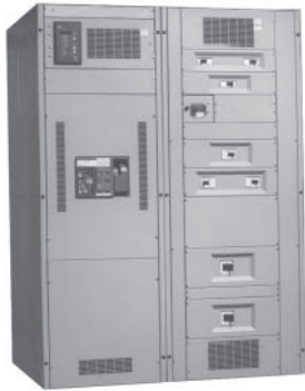
Front View—Circuit Breakers
